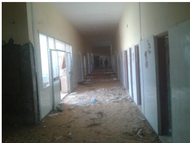
The Alberkat Clinic Centre in Ghat before the rehabilitation. ©UNDP Libya
