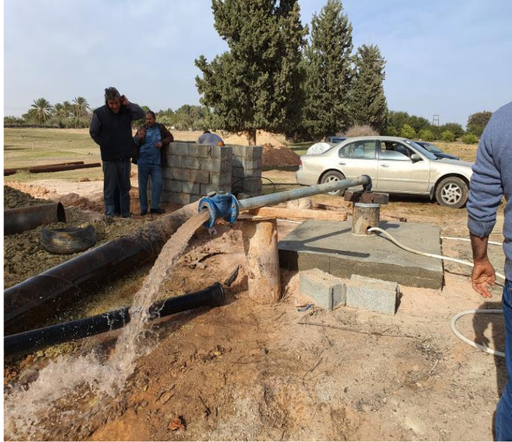
Excavation and equipment of 4 wells for drinking water in Garabulli. ©UNDP Libya
