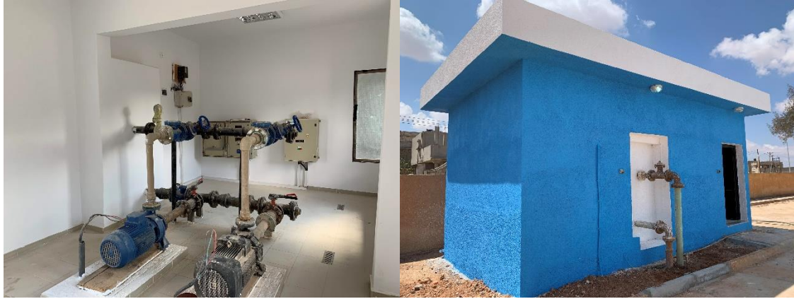
Exterior and interior of the Water Pump Station after rehabilitation in Benghazi. ©UNDP Libya
