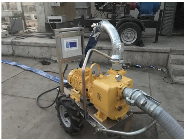
UNDP supplies the Municipality of Sebha with four sewage pumps. ©UNDP Libya
